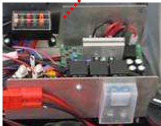
Main electrical board and fuses
